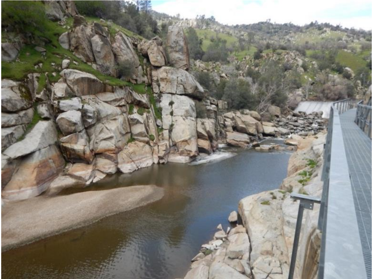
Photo A-6. Looking upstream at the Diversion Dam (spilling) from the slide gate valve house.
