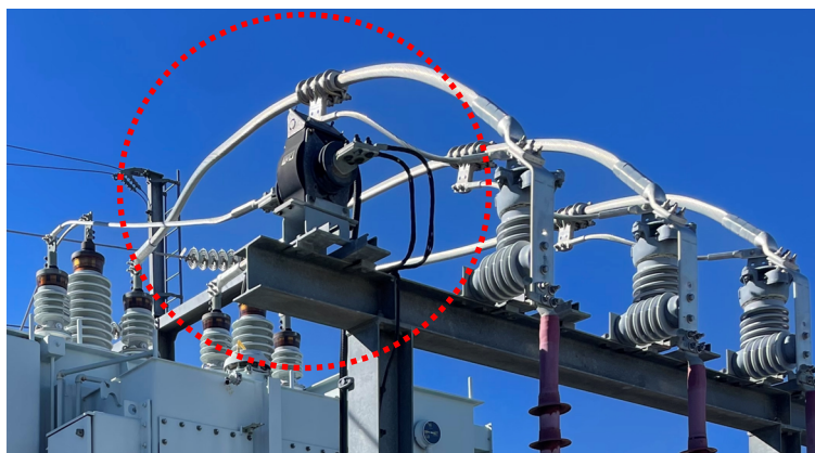
Figure 50: Typical Current Transformer on the neutral of a substation transformer
