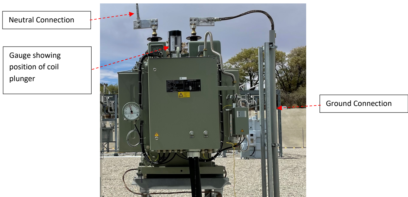
Figure 48: Overview of arc suppression coil at Arrowhead substation
