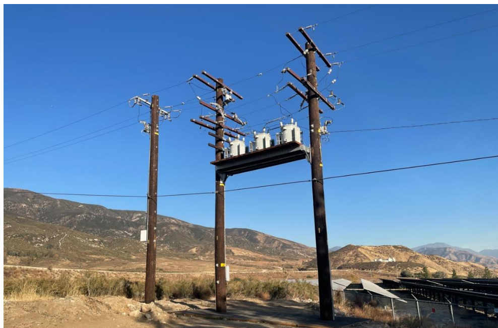
Figure 62 Isolation Transformer Installed on the Calstate Circuit
