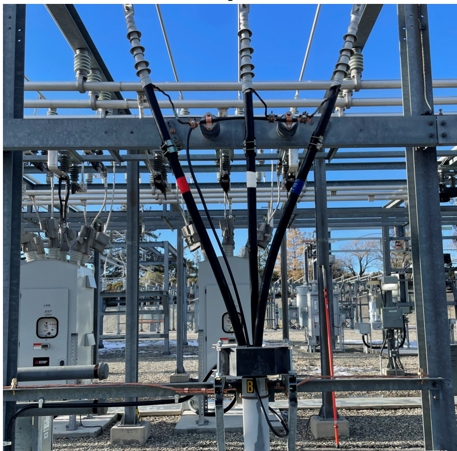
Figure 51: A zero sequence current transformer around all three phases of a distribution line
