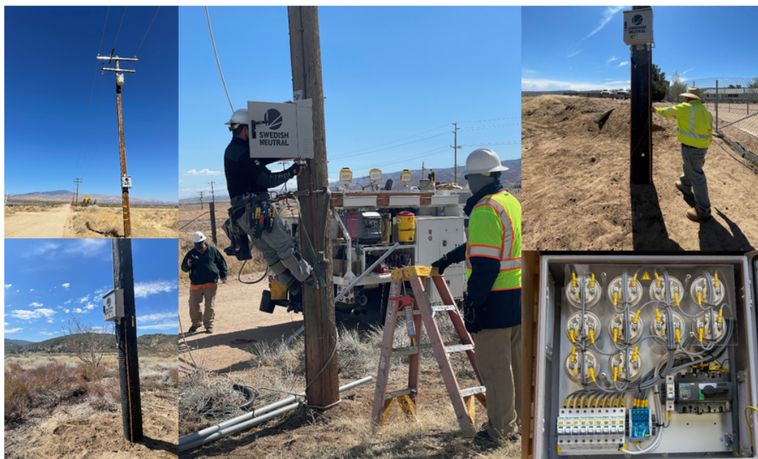
Figure 23: Capacitive Balancing Units Installations
