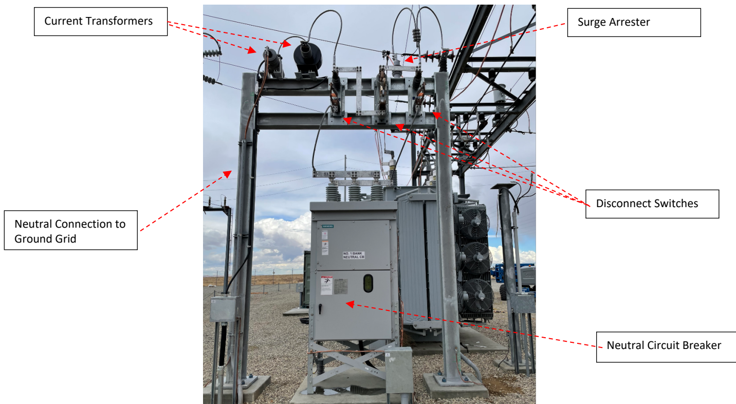
Figure 15: Neutral Circuit Breaker for Ground Fault Neutralizer in Initial Configuration
