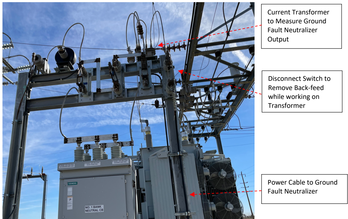
Figure 17: Ground Fault Neutralizer Connection Moved to Main 66/12kV Power Transformer Neutral
