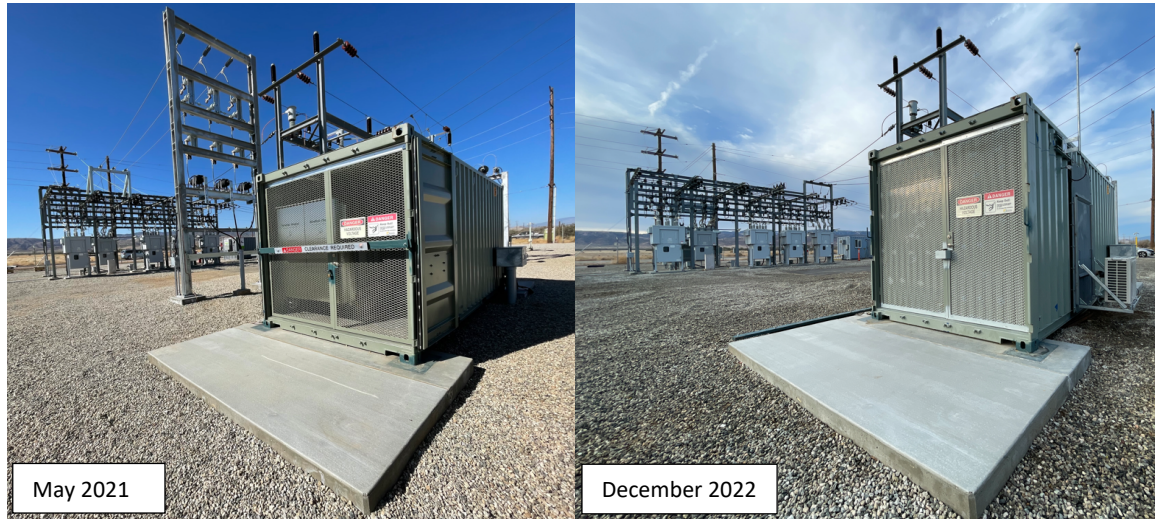
Figure 19: The 12kV Connection into Ground Fault Neutralizer removed in Q4 2022 rebuild
